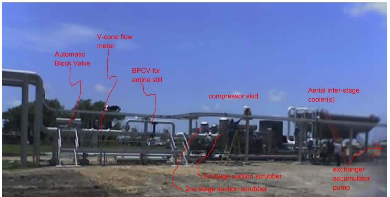
Figure 1 and Figure 2 are photographs taken from AGI Compressor sites that Trimeric designed.
