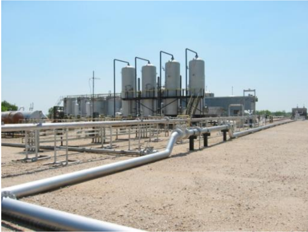
Figure 2 Tower-Based Scavenger Installation in South Texas
