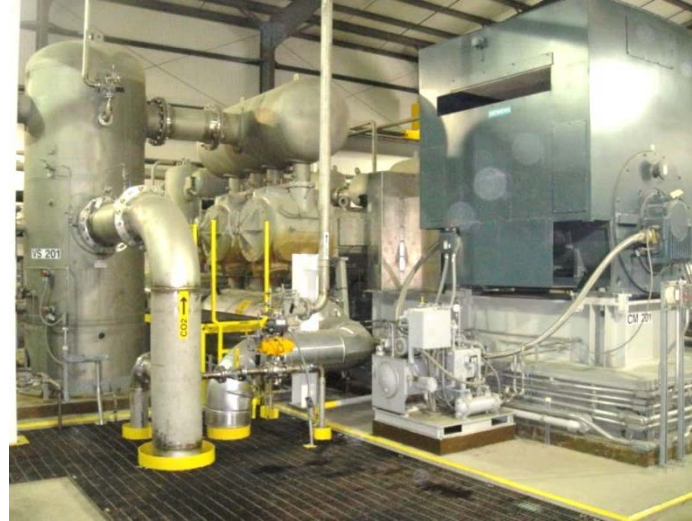
ADM Decatur / MGSC 400,000 tonne/year CCS Plant 3,250 hp (2,425 kW), 4-Stage, Reciprocating Compressors (x 2)
