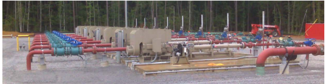
Centrifugal Pumps at CO 2 Pipeline Booster Station
