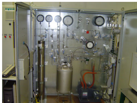
Figure 14. Gas Feeding System
