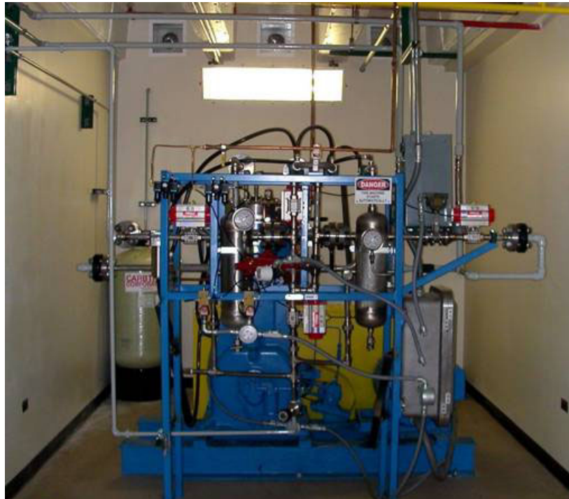
Figure 6. Booster Compressor and Ancillary Equipment
