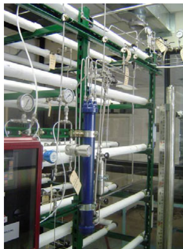
Figure 11. Sampling Lines to H 2 S Analyzer
