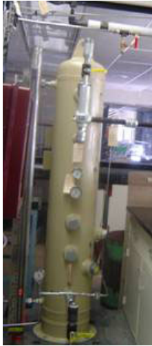
Figure 7. Fresh Scavenger Storage Tank
