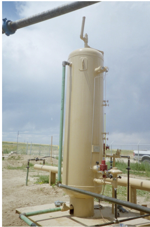
Figure 8 - 36” Diameter, 8’ Seam-to-Seam Surge Bottle
