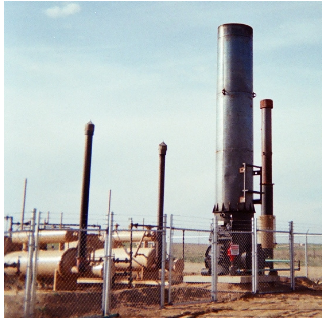
Figure 4 – 48” Burner (Largest Stack Shown in Picture)
