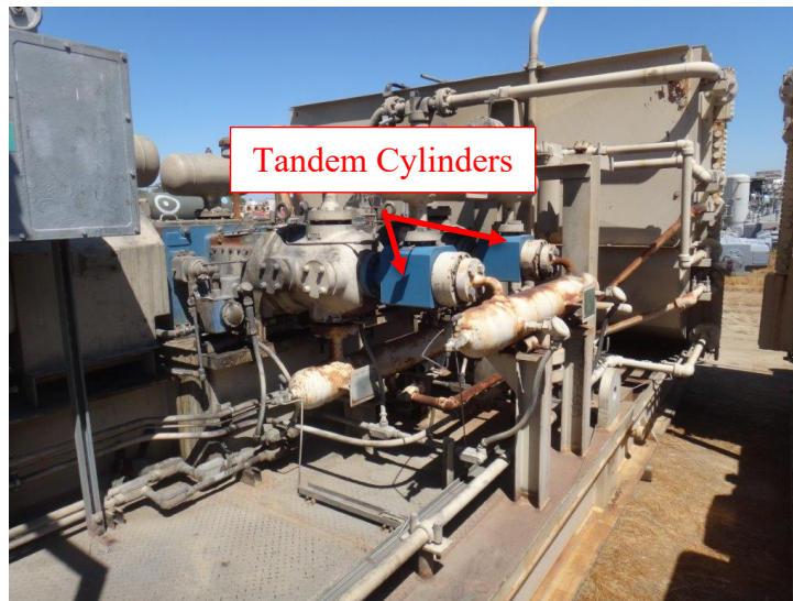
Figure 4. Example Tandem Cylinders on Reciprocating Compressor.
