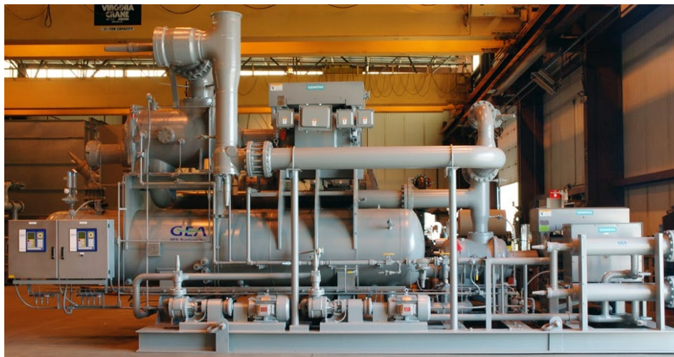
Figure 6. Typical Oil-Flooded Screw Compressor Skid (Courtesy of GEA FES).
