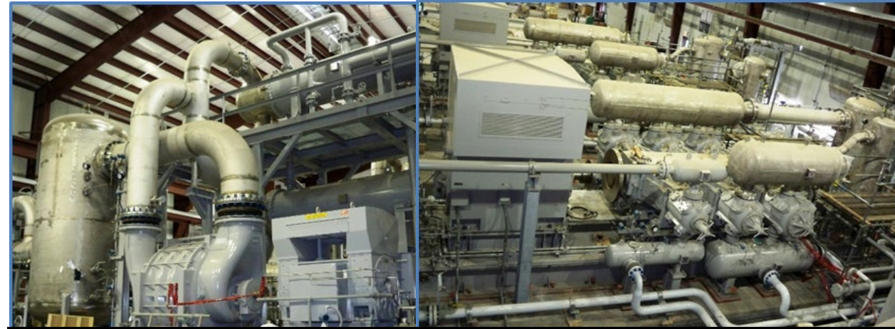
1 MM tonne/yr facility design. Blower (left) and compressor (right) skids
