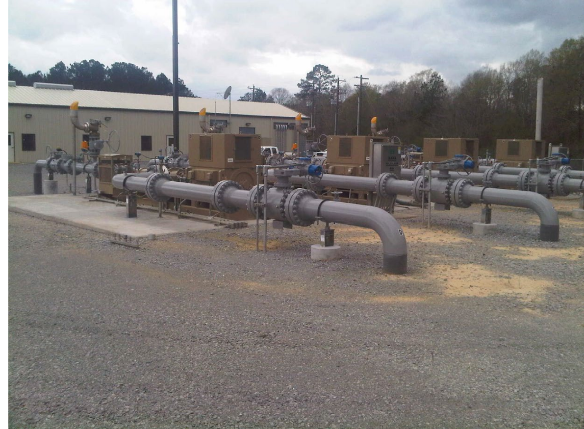
Pumps at 1,425 tph CO 2 Pipeline Booster Pump Station
