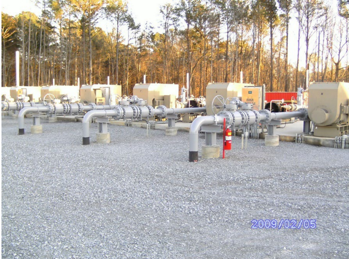
Pumps at 1,750 tph CO 2 Pipeline Booster Pump Station
