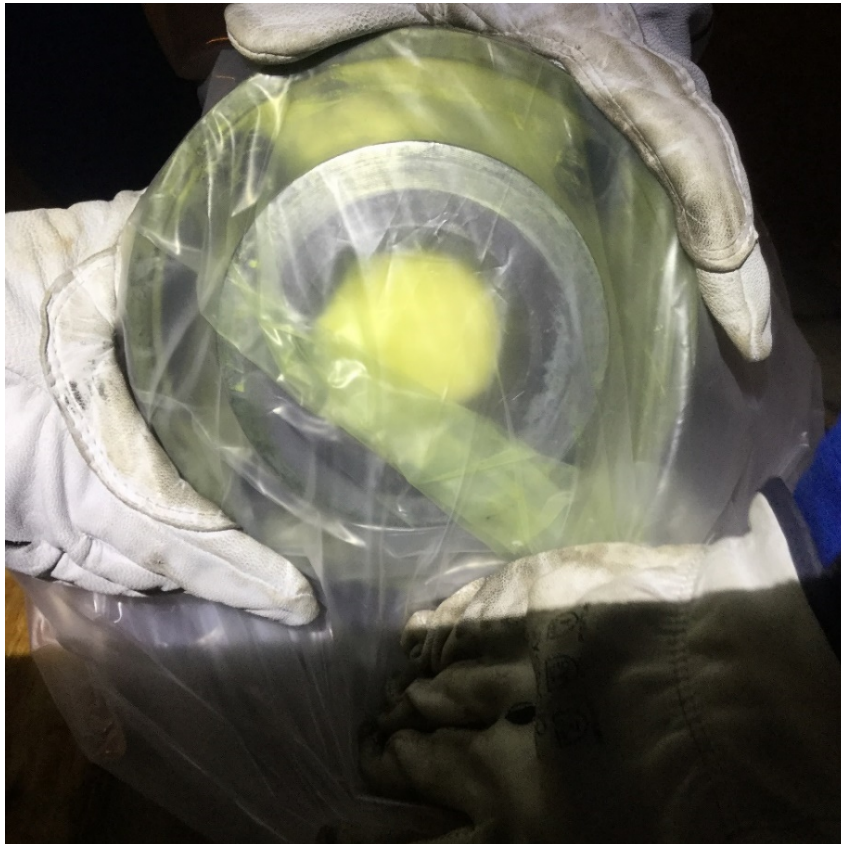
Figure 2. PRV Inlet Piping on Headspace of Sour Water Stripper (large gulf coast refinery).
