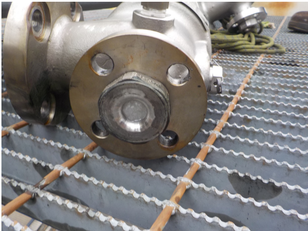
Figure 4. PRV Inlet Piping on Headspace of Sour Water Stripper (unidentified refinery).
