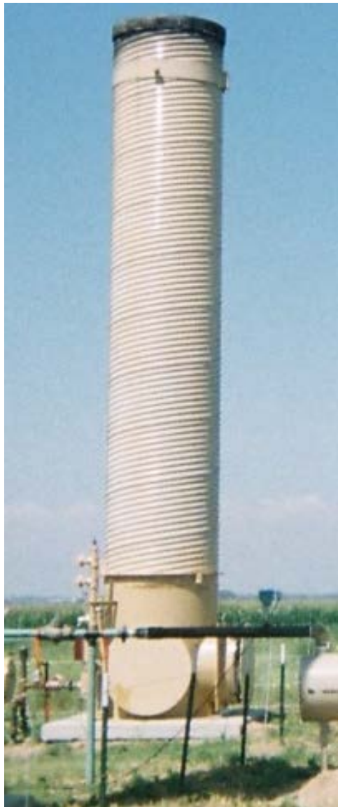
Figure 6 – Picture of Enclosed Flare
