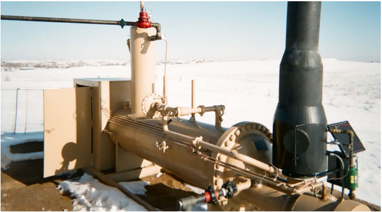
Figure 2 – Picture of Single Stage Production Separator
