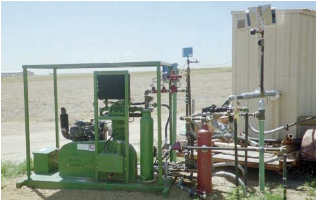
Figure 7 – Picture of Two Stage Reciprocating Compressor VRU
