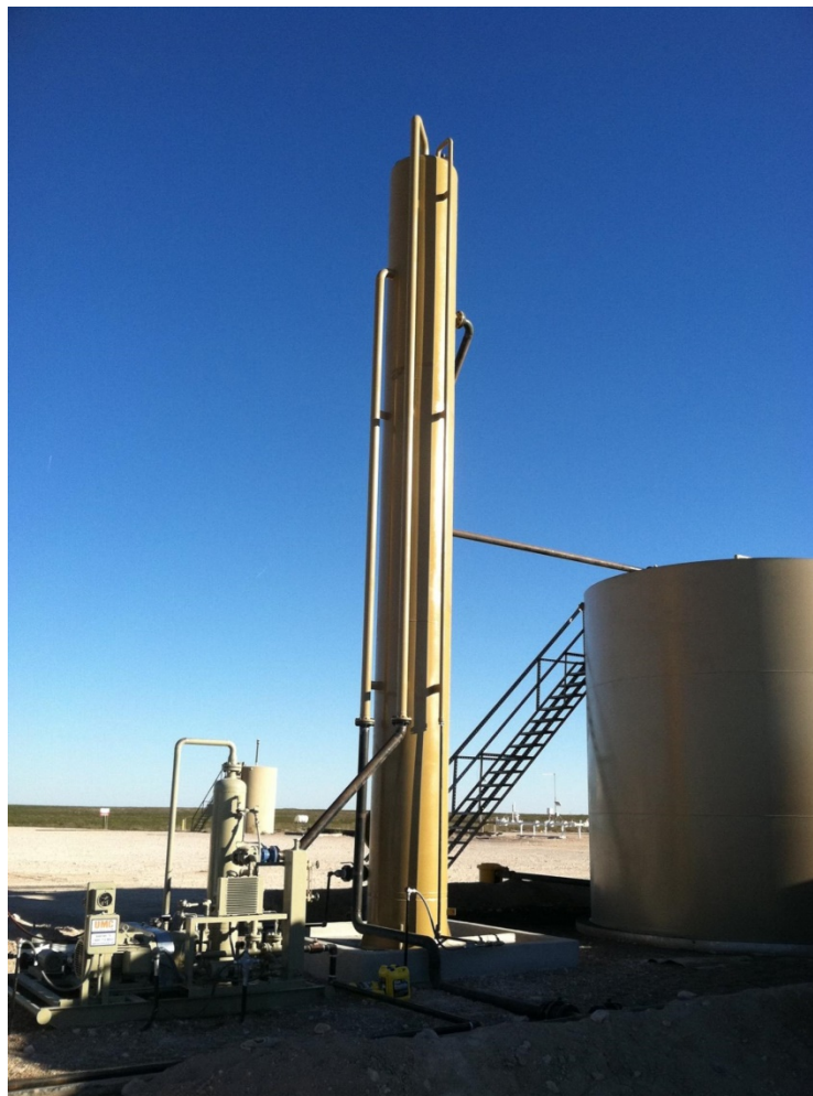
Figure 13 – Picture of Vapor Recovery Tower. Photograph courtesy of Reset Energy.
